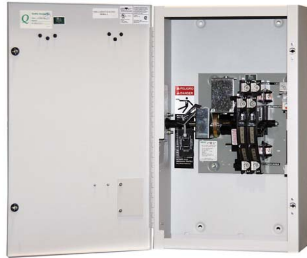
185 Manual Transfer Switch Door Open
